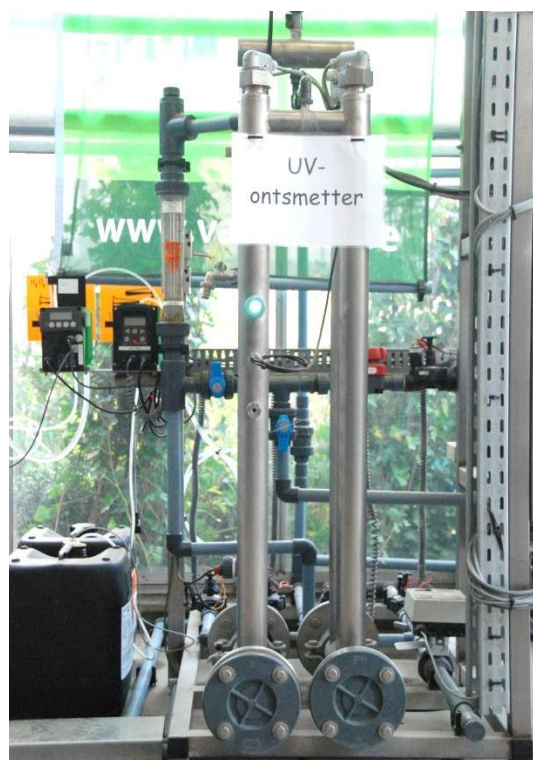
Figure 6.2: Front image of the UV/H 2 O 2 reactor that was used
